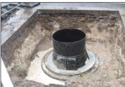
9.) Filling the gap between PE-chamber DN 800 and DN 1000 concrete manhole with filling mortar
