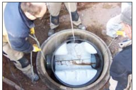
5.) Adapt the prefabricated channell with PE socket and place it into the chamber bottom
