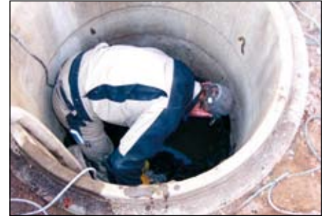
2.) Remove climbing steps, pry berm and flume, dewatering, set the over-pumping operation
